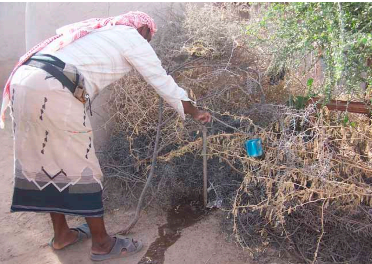
Yard connection in Yemen
