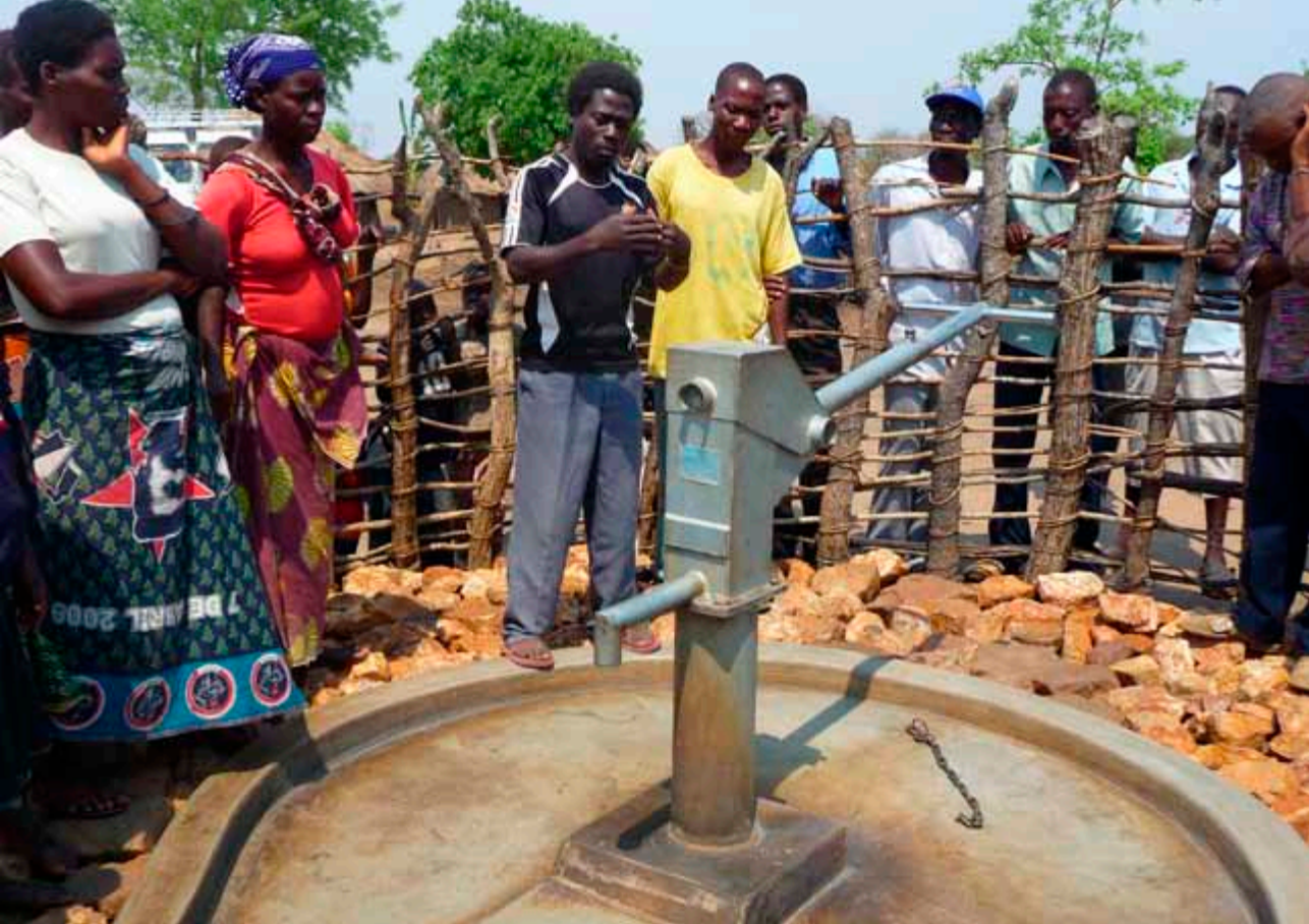
Communal waterpoint in Mozambique
